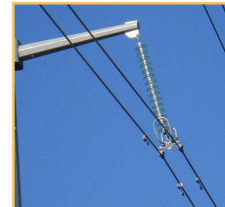
BC Hydro - North Transmission Line (NTL) 287kV twin bundle 325km Line Hardware & fittings and damping system.
