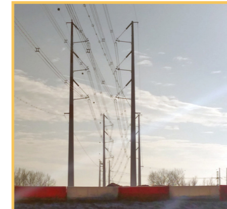
Tennet project doetinchen - wesel Wintrack project line 380kV spacer dampers.
